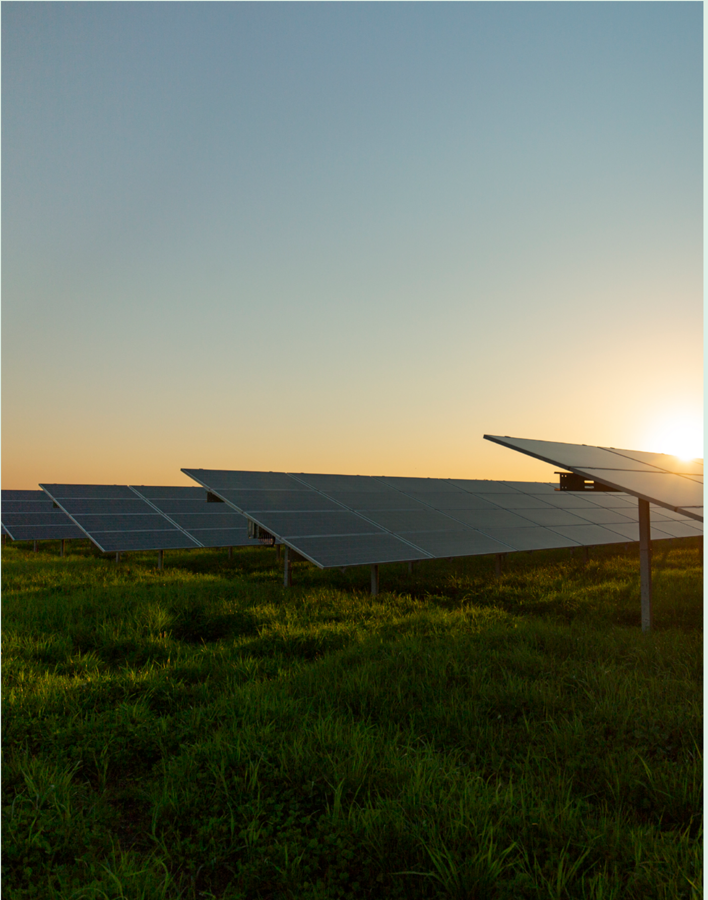
NRGi Solcellepark Nees
